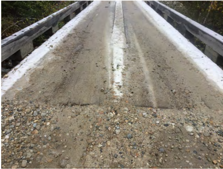
Minor wear on planks
